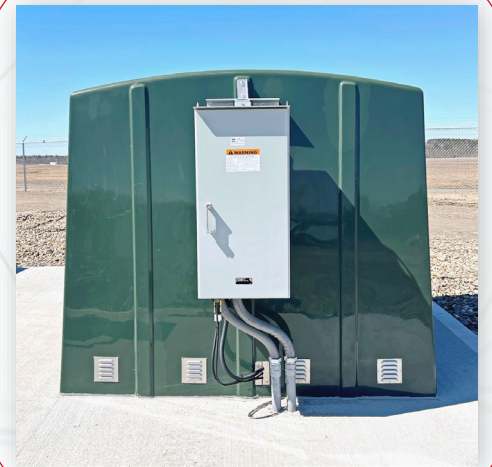
Recloser control module installed on the enclosure
