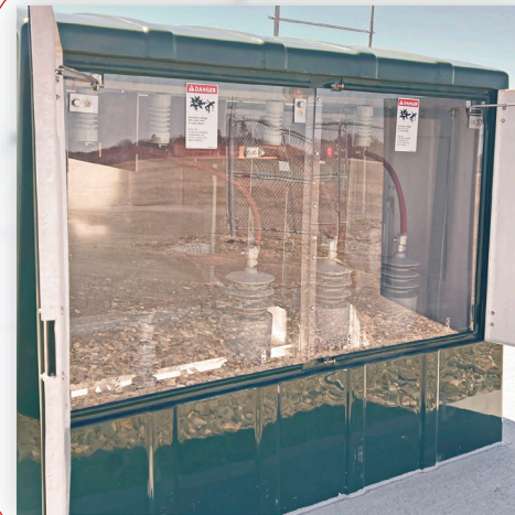
Clear Lexan inner door on reclosure side only
